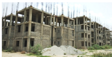
Picture 3: Project at Poothkhurd Phase-III lying incomplete and idle since January 2018
